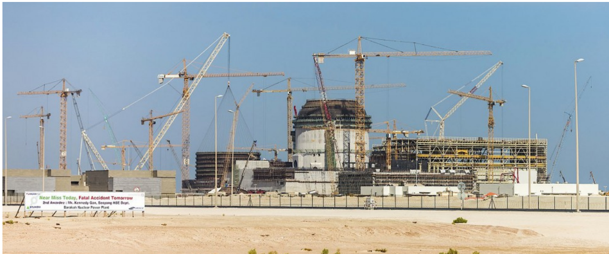
Unit one is now 55% complete, and the whole project more than 35% complete. The aim is to commission the first reactor in 2017 with three more plants coming online each year to 2020. (credit: ENEC)
