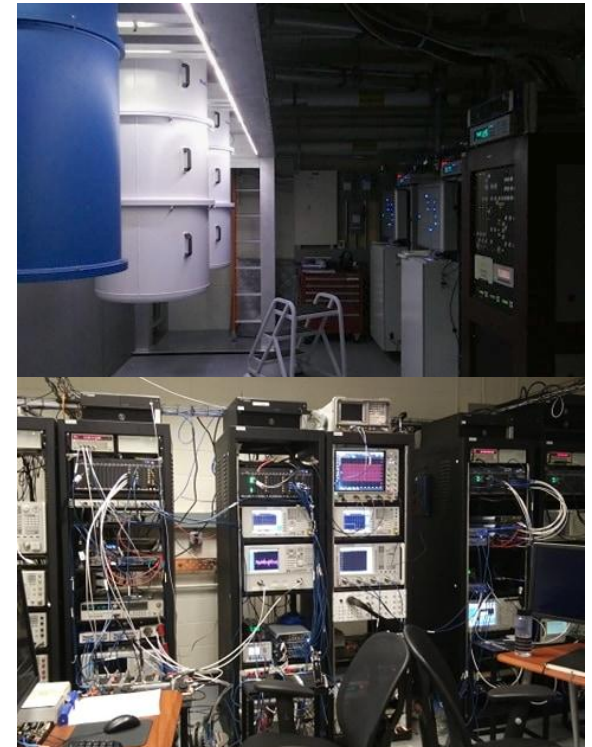
Lab Measurement Racks
