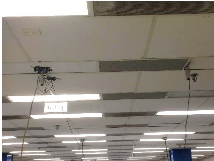
Figure 2 Two NTSC Camera Setup. The two cameras were installed in the ceiling using electrical tape, and they were connected to the power sources and Labkits using very long cables.
