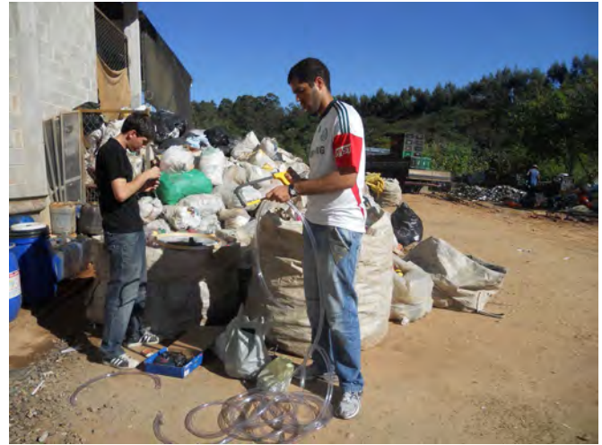
Walter Volpini and Denis Ferreira installing a waste vegetable oil filtration system at ARES Cooperative. Photo by Marta Marella
