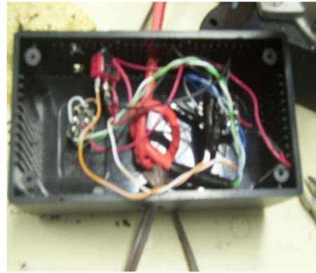
B: Control box with completed thruster switches
