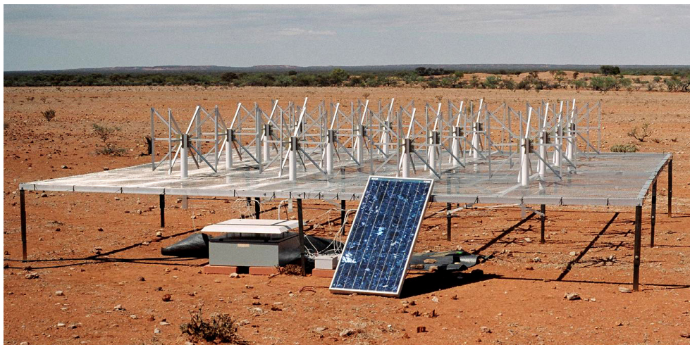
Figure 3. The first completed antenna station with beamformer box and battery-backed solar power supply deployed at Mileura, Western Australia.
