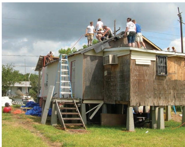
With a PSC grant, MIT student volunteers spent spring break repairing and rebuilding a house in Houma, LA, as part of the Lift House Project.
