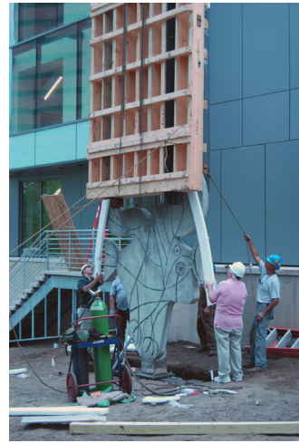
Workers installing Pablo Picasso's sculpture Figure découpée in its new location at MIT's Sloan School of Management.
