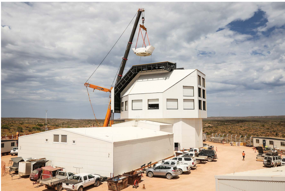
Figure 2. The Space Surveillance Telescope mount installation is under way in the newly completed enclosure in northwestern Australia.
