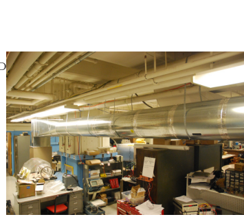
Fig. 12. View of ducting apparatus.
