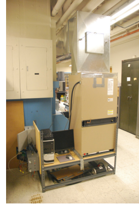
Fig. 10. Picture of the overall air handler apparatus and attached duct system.
