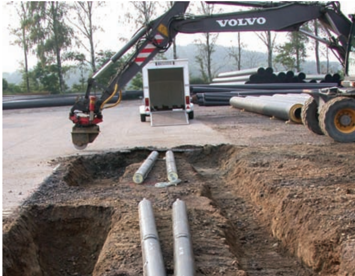
District Heating/Cooling Network Installation > Piping is installed for a district heating and cooling network in Sweden. Pipes must be heavily insulated and buried underground. Source: SP Technical Research Institute of Sweden 2008.
