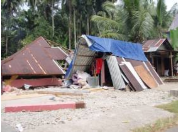
Temporary shelters built next to their damaged house made from reclaimed material.
