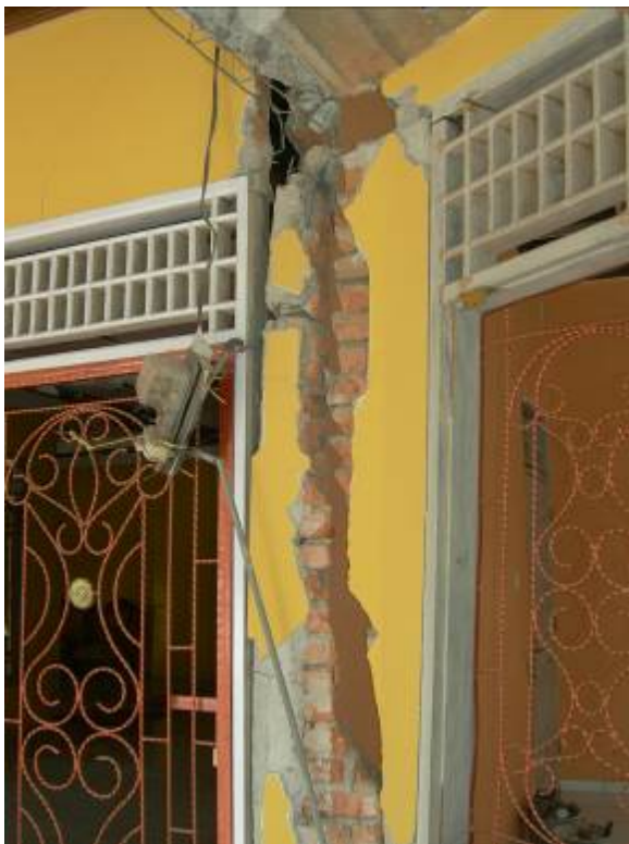
Size of structural columns too small and low quality of re-enforcement bars.
