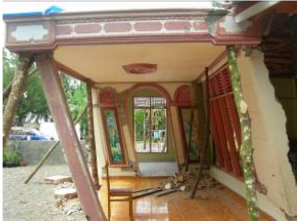
Lack of lateral bracing, dangerous structure.
