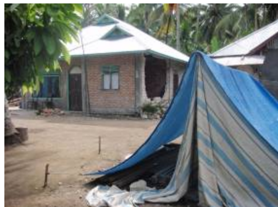
Tents made next to the damaged house
