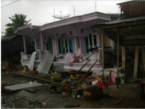
Entire ground floor collapsed.
