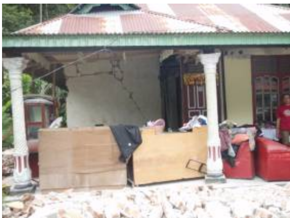
Living under damaged veranda
