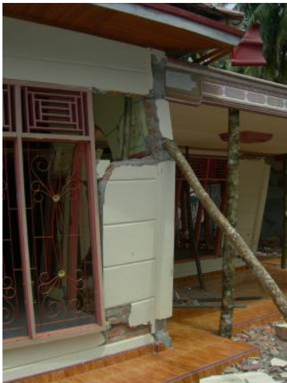
Dangerous structures left and owners put supports to avoid collapse.
