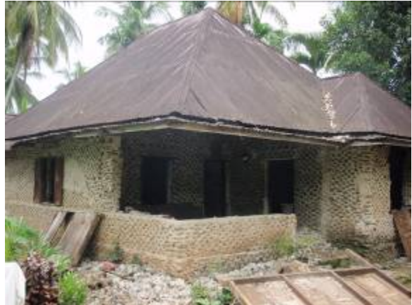
Weakness in corners without structural columns
