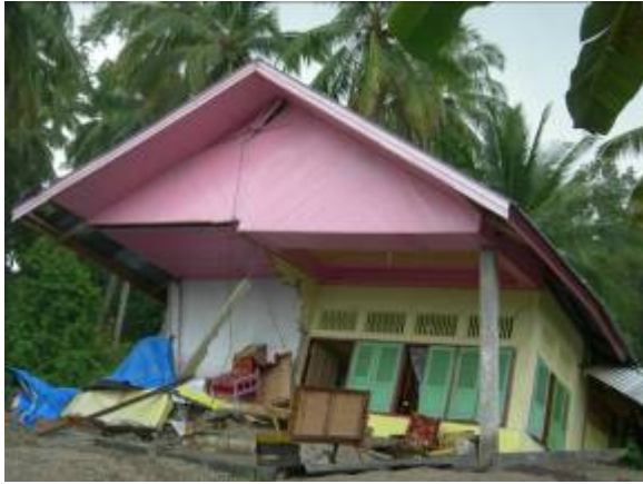
Land movement, causing sedimentation to the foundations, relocation and tenure issues may become important.
