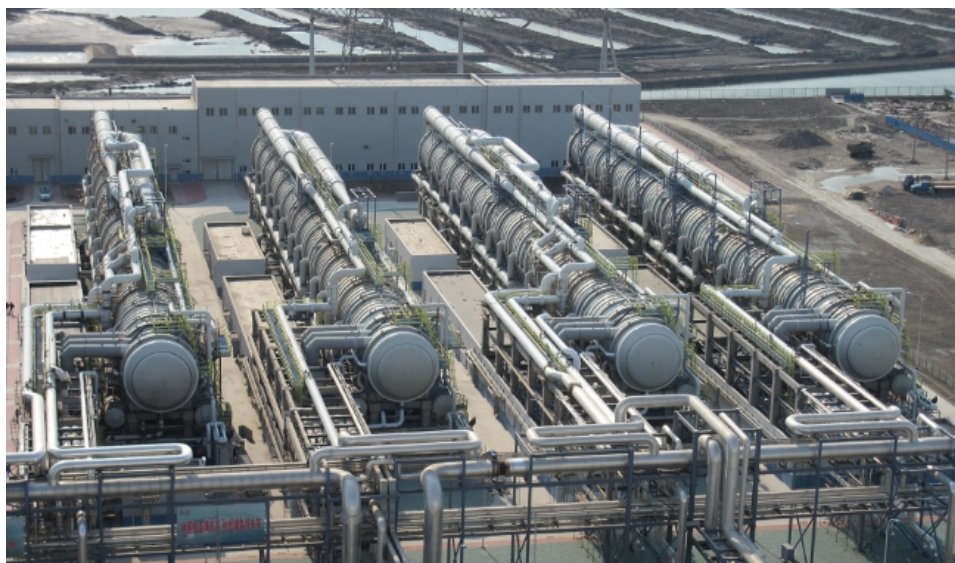
IDE Technologies' 200,000 m3/day plant in Tianjin, China is one of the world's largest MED desalination facilities
