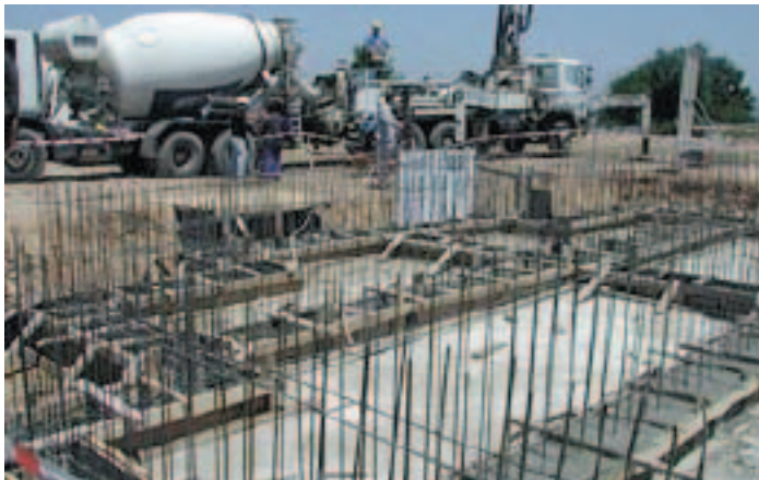
The "groundbreaking" ceremony for Berikoy was actually a "concrete-shoveling" into the forms that had been laid for the foundations of the first houses.
