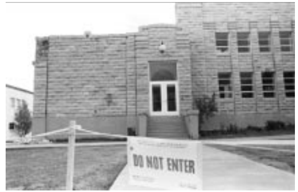
Figure 4. The separated façade of a Challis, ID high school following the Borah Peak earthquake of 1983. Photo by Sue Villard, courtesy of The Challis Messenger.
