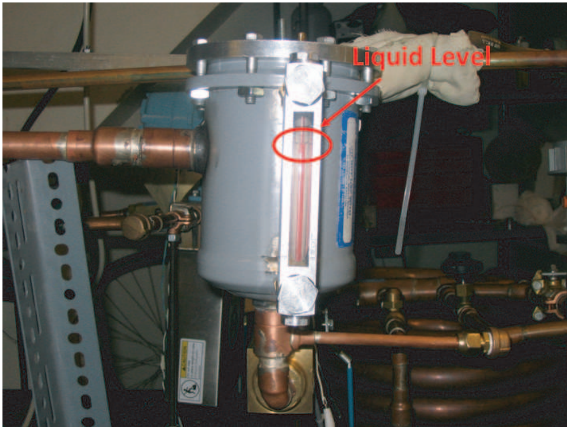
Figure 2-5: New filter drier with liquid level indicator.
