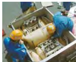
Placing a capacitor in a container
