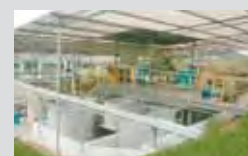
Waste treatment facilities (after improvement)
