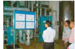
Exhaust heat recovery system of Beijing Matsushita Color CRT Co., Ltd.
