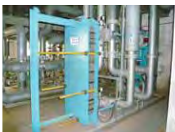
Waste heat recovery system
