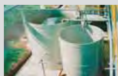
Waste treatment facilities (before improvement)
