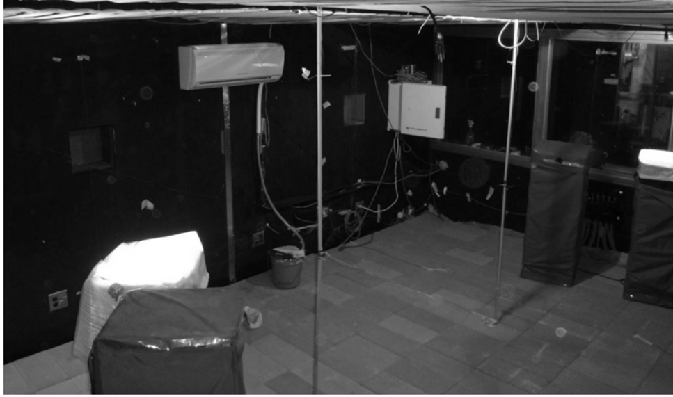
Figure 4. Test office chamber with concrete radiant floor, simulated internal loads, and a conventional split-system air conditioner indoor unit (the base case system)
