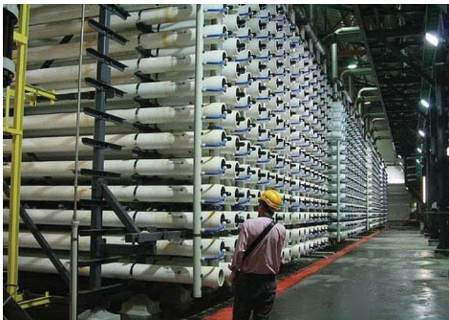
Ashkelon desalination plant
