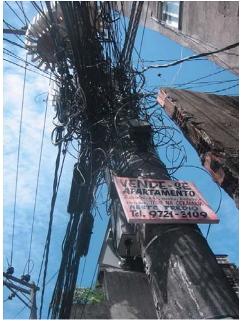
Figure 6. Favela homes and businesses connect to public utilities by fazendo um gato , or making an illegal connection to main lines or one legitimate subscriber.
