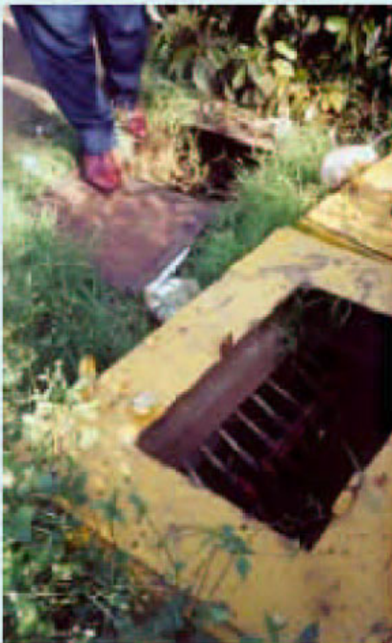
A metered manifold box.
