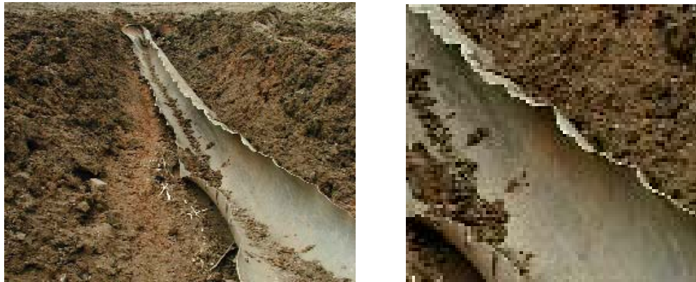
Unzipping a pipe leaves a wavy crack edge
