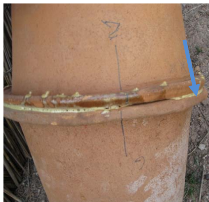
Figure 6-8 Holes in the Seal Due to Lack of Gorilla Glue
