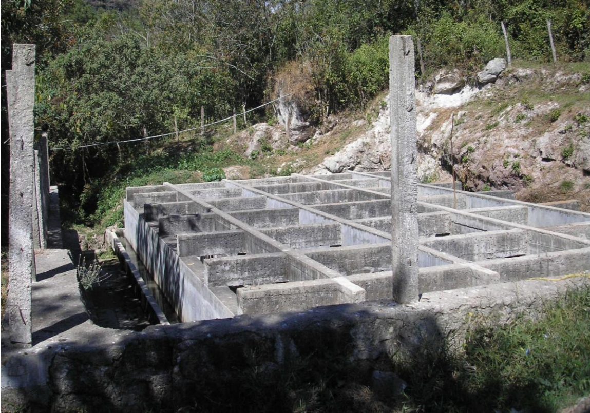
Figure 5 Marcala Imhoff Tank
