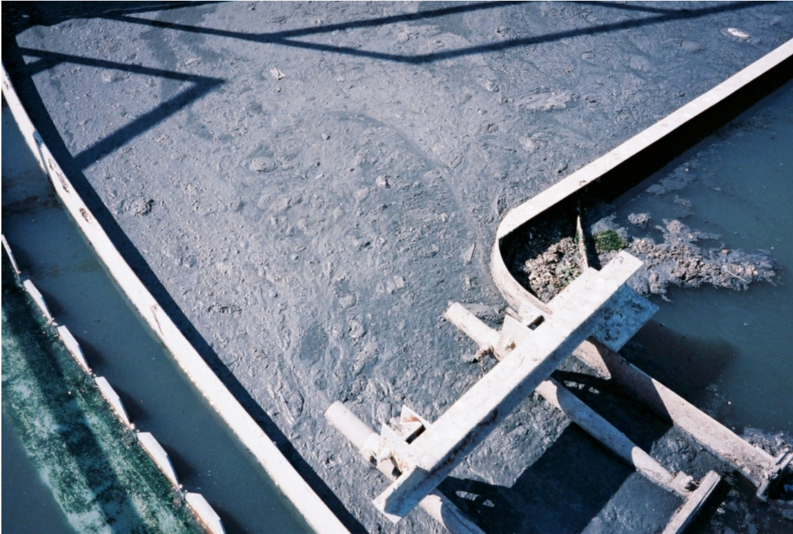
FIGURE 6: FLOATING SLUDGE AT VEGA BAJA
