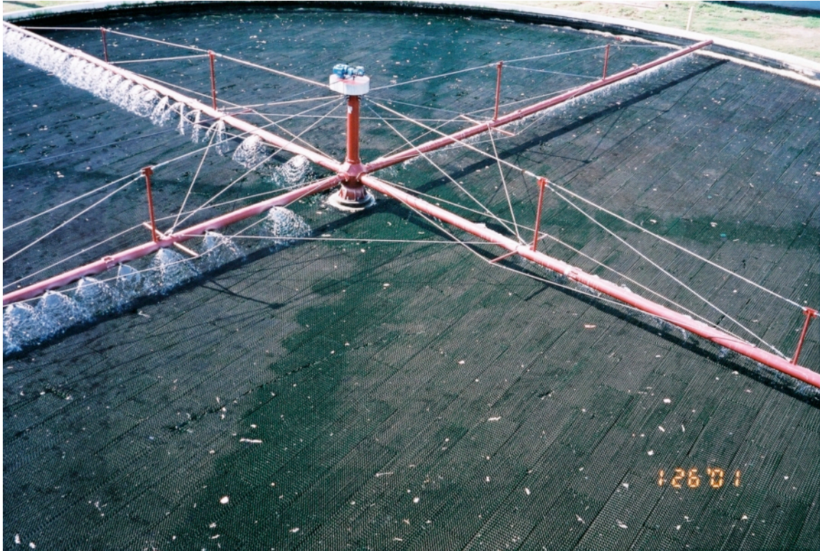
FIGURE 8: DRIED OUT TRICKLING FILTER AT FAJARDO – THE DARK LINES ARE THE NORMAL COLOR OF THE TRICKLING FILTER AND ARE WHERE THE ARMS WERE STOPPED FOR MAINTENANCE ON THE PREVIOUS DAY.
