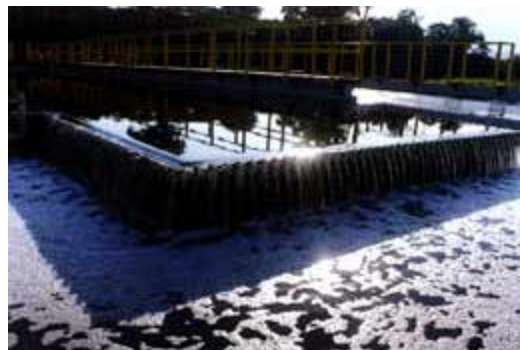
Figure 1-6: Detail of the CEPT tanks at Riviera de São Lourenço (Source: http://www.rivieradesaolourenco.com )
