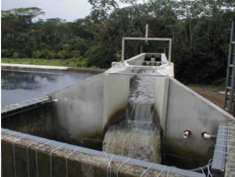
Figure 8-3 Chemical Dosing System and Ultrasonic Flow Meter at Riviera
