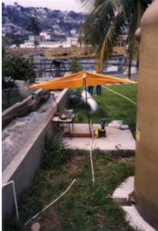
Figure 6-2 Chemical Dosing Area at ETIG
