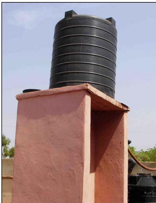
Figure 30: Source Water From Elevated Tank in Tamale
