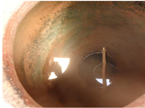
Figure 62 View Inside a Water Vessel Reserved for Clean Tap Water
