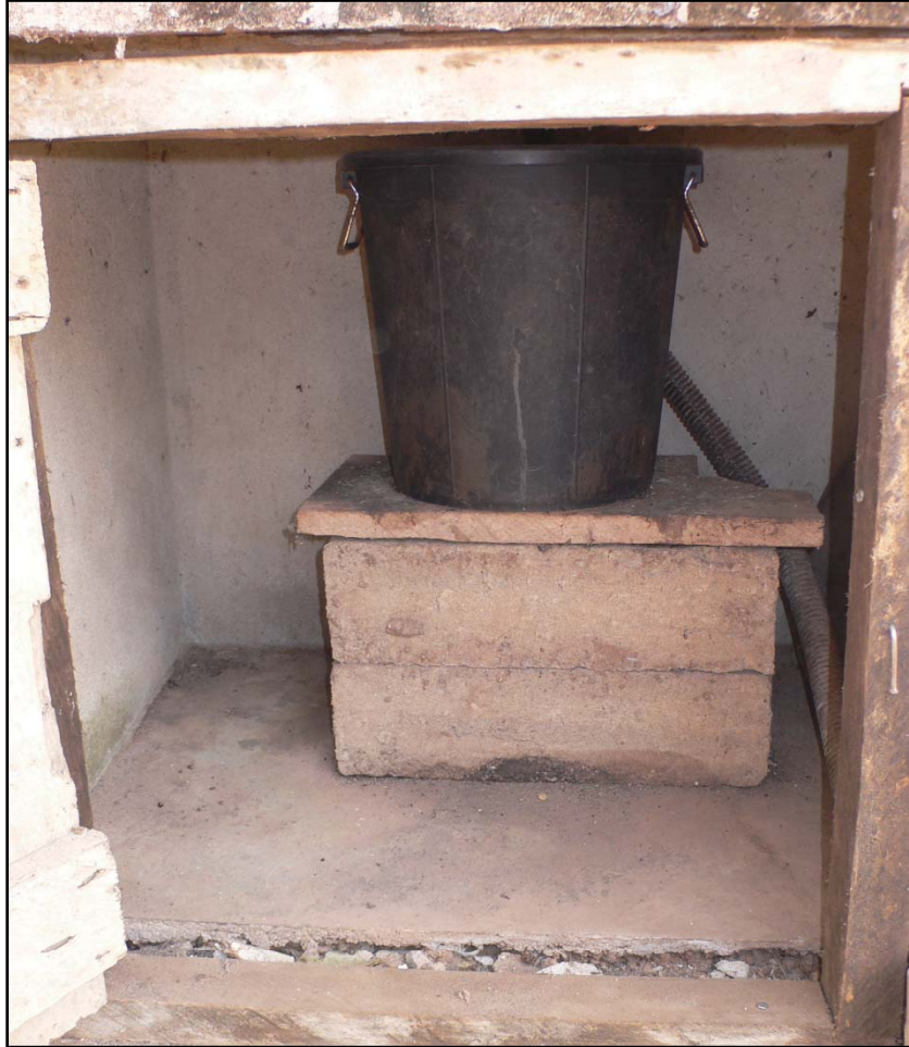
Figure 5-8 Removal Bucket at the back of the EcoSan latrine and urine diverting pipe
