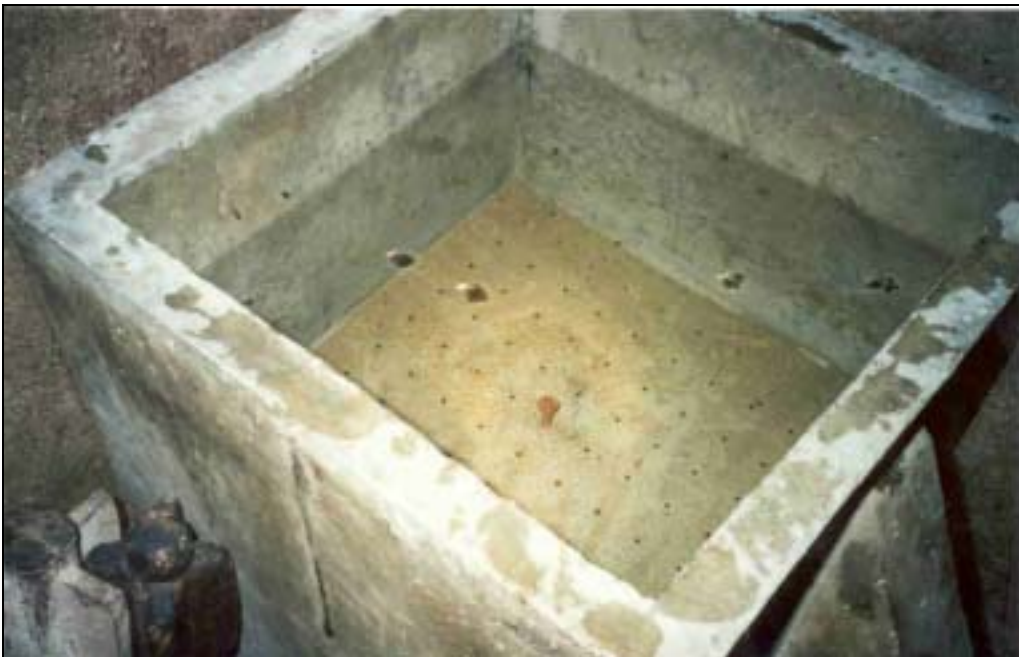
Figure 37: Water level at rest more than 5cm above the topmost sand level.
