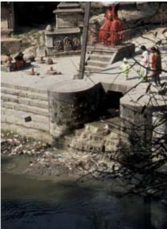
Figure 25: Picture of the sewage outfall at the Gujeshwari Temple.
