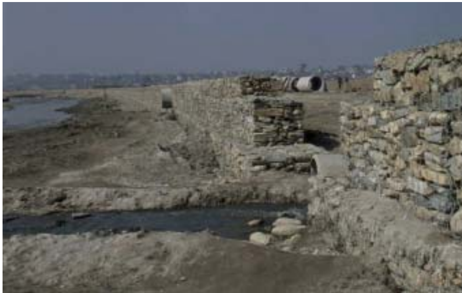
Figure 24: Picture of a large outfall discharging raw sewage into the Bagmati River.
