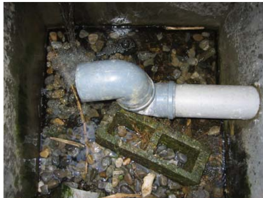
Figure 5.12: Effluent of the Constructed Wetland System
