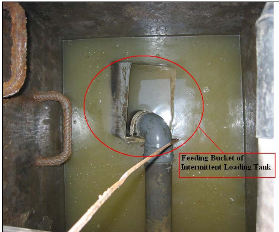
Figure 6.9: Feeding Bucket of Intermittent Loading Tank
