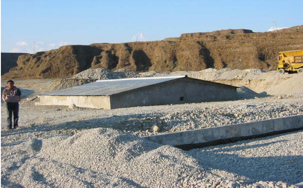
Figure 5.15: Septage Settlement Tank
