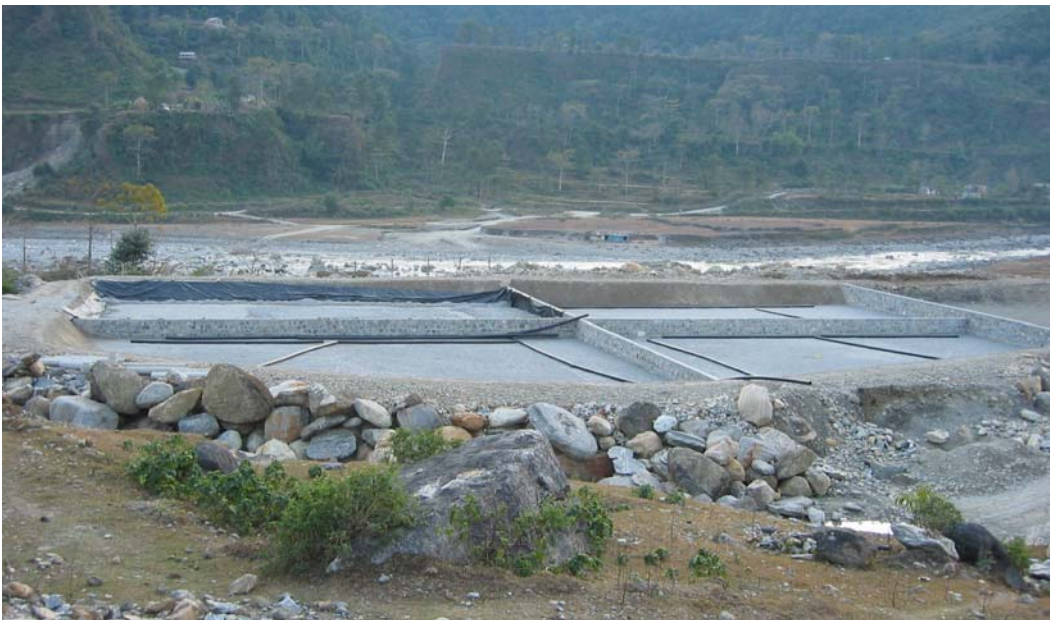
Figure 5.20: Vertical Flow Bed at Kathmandu
