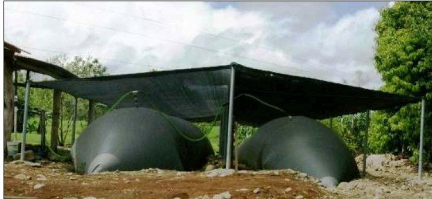
Polyethylene tube biodigester
