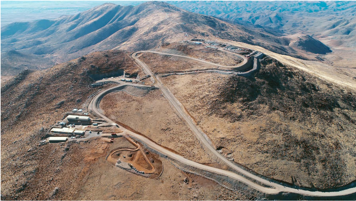
Construction site for the 25.4-meter Giant Magellan Telescope, on Las Campanas Peak, Chile. Dome excavation trench is visible on the summit, with residences at lower left and laboratory building site at center. The 6.5-meter Magellan Telescopes, currently in use by MIT Kavli Institute researchers, are visible on the adjacent peak along the ridge access road, at the top center of the photo. Credit: Giant Magellan Telescope Organization.
