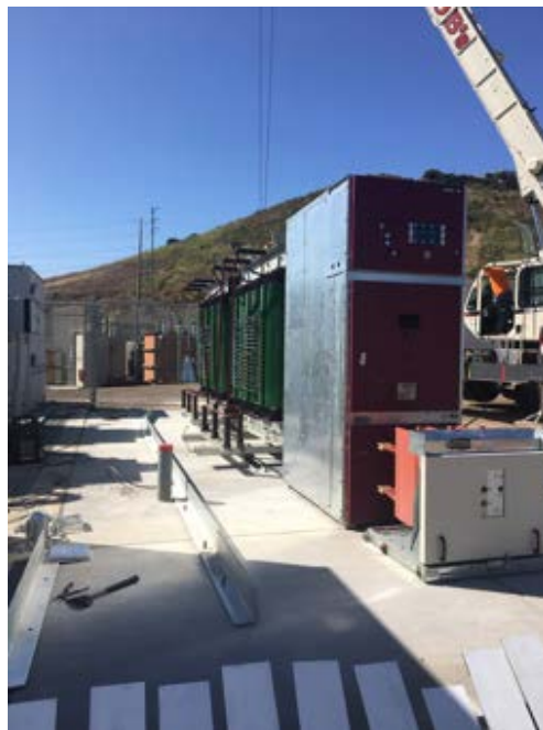
Figure 3. DIII-D high-voltage power supply.
