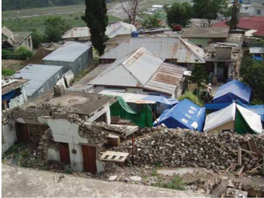
Picture 7. Western edge of residential area near the river. Flat terrain. Brick building almost completely collapsed. Minimal structural damage to metal buildings. 10-30 years old.
