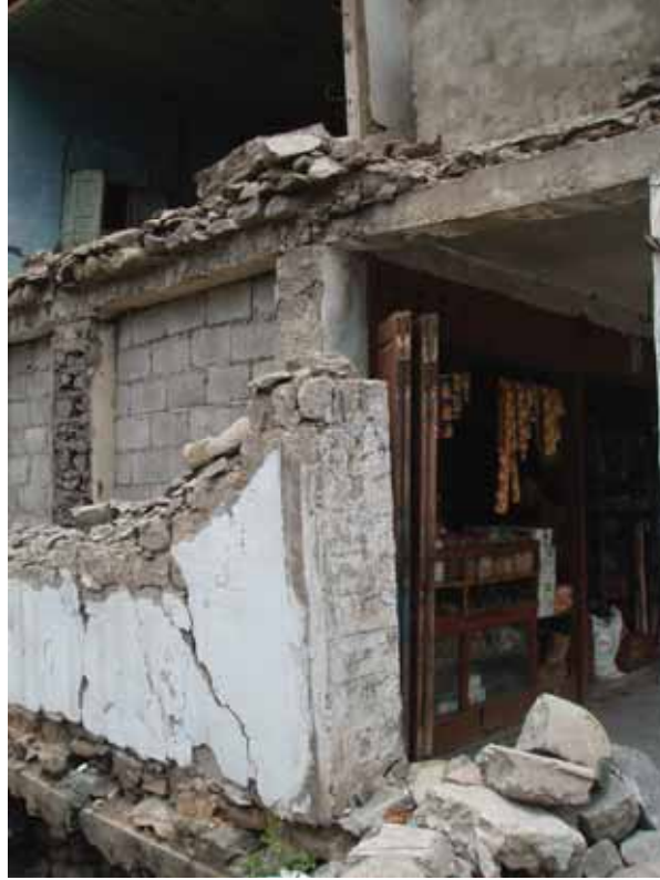
Picture 5. Center of residential area. Collapsed front walls were stacked brick and stone mixed with cement and mortar. Remaining structural walls were all intact. Gently sloping terrain. 10-30 years old.
