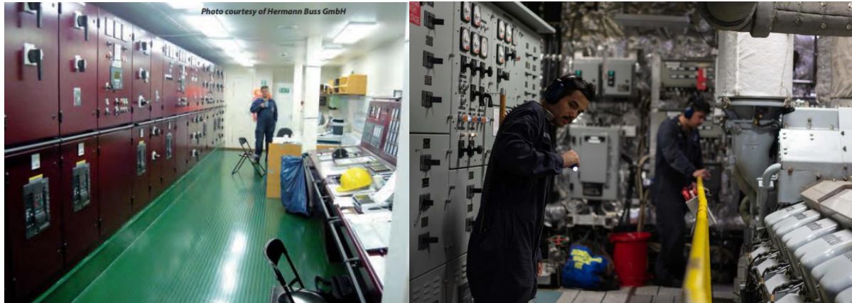
Figure 6-1: A switchboard in a commercial ship (left) [85] and switchboard on USS Jackson (right) [86]
