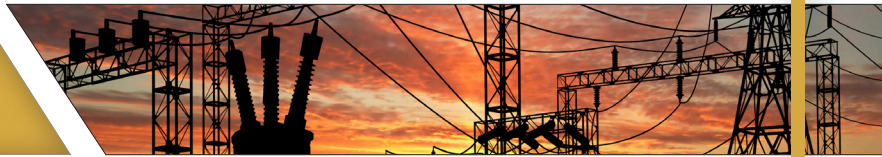
Transformer and Sunset | Electric Companies 2013
