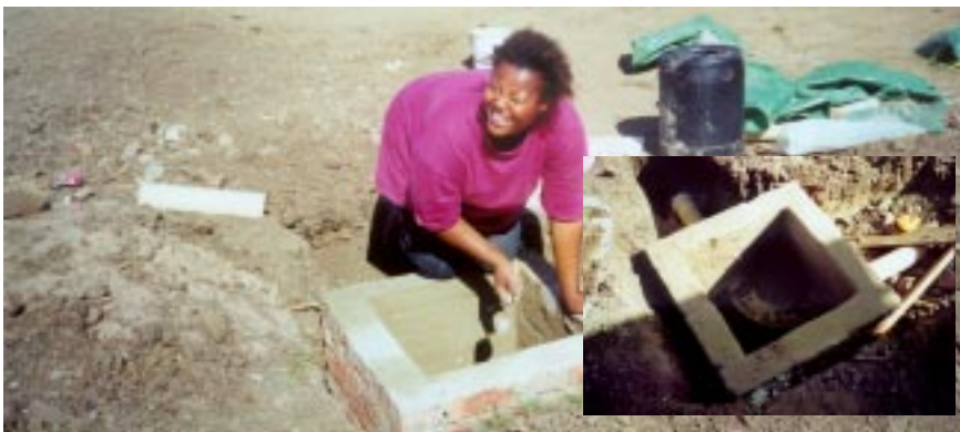
Condominial Sewerage Systems: Community members build and maintain a network using small pipe diameters.
